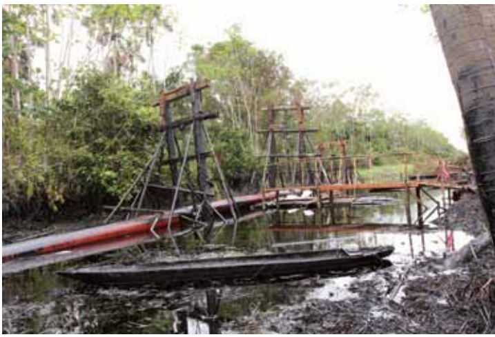
Damaged section of pipeline is raised above water level using pulleys mounted on pylons. (Photo by Barbara Fraser)
